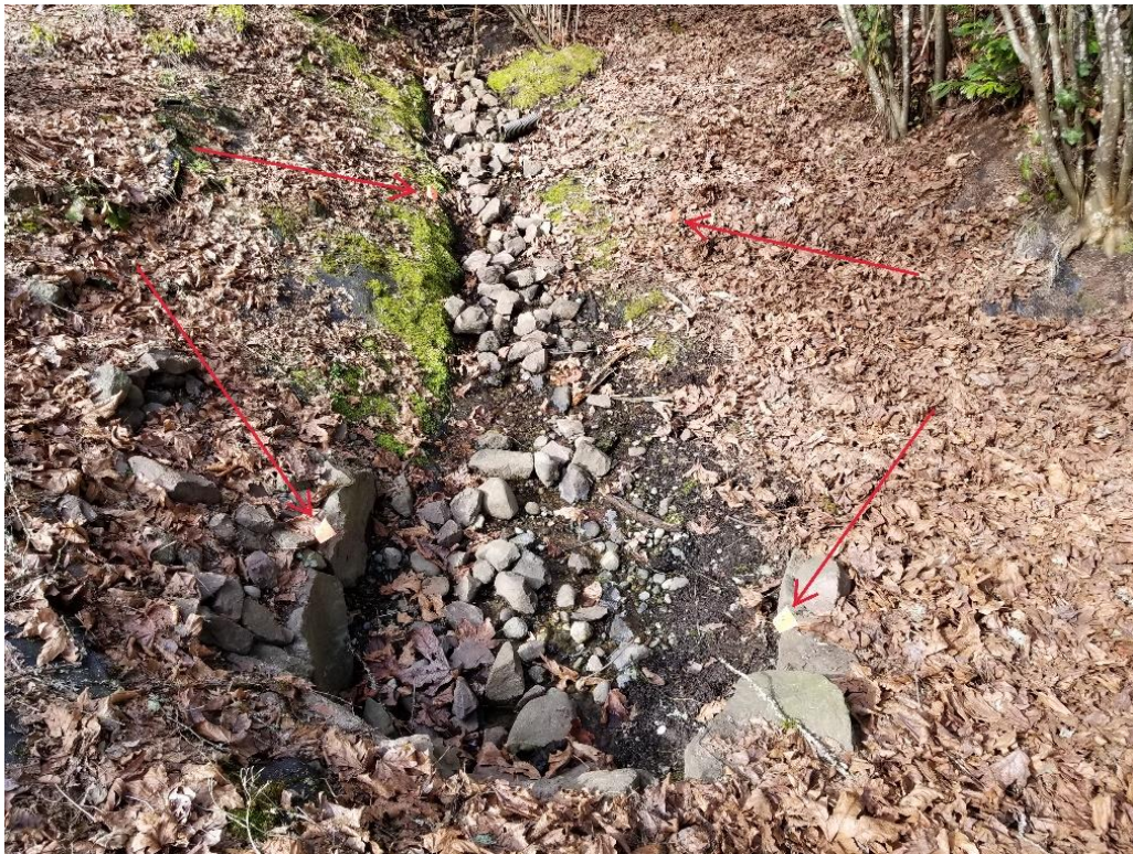
Photo 10—Delineated OHWM, facing west. Red arrows show location of visible pin flags.
